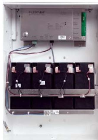
Front view MPS48-7 shown with batteries and AC service installed
